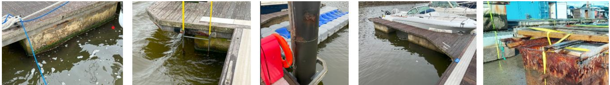
Images of the pontoons highlight the likely degradation of the fuel jetty when recently removed. Image source: Blue Sea Consulting LLP 2023
